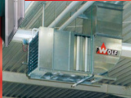
Air Inlet Plant
