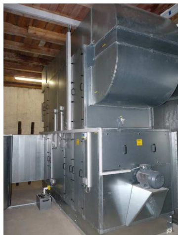
Fig. 3: Heat exchanger with condensate recovery
